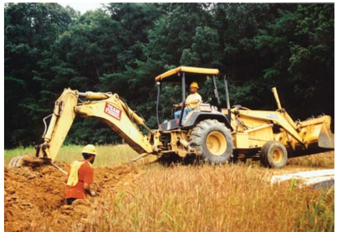
Danny Pyles backhoes a section of a trench for Dominion Power in Fredericksburg, Virginia.
